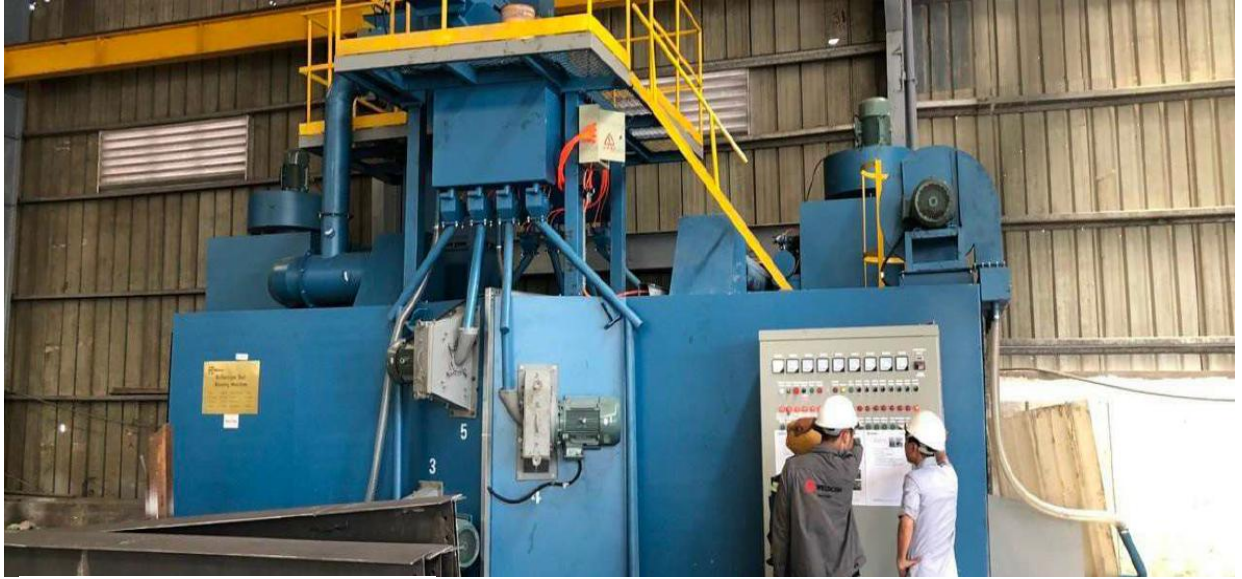
SHOT BLASTING LINE
